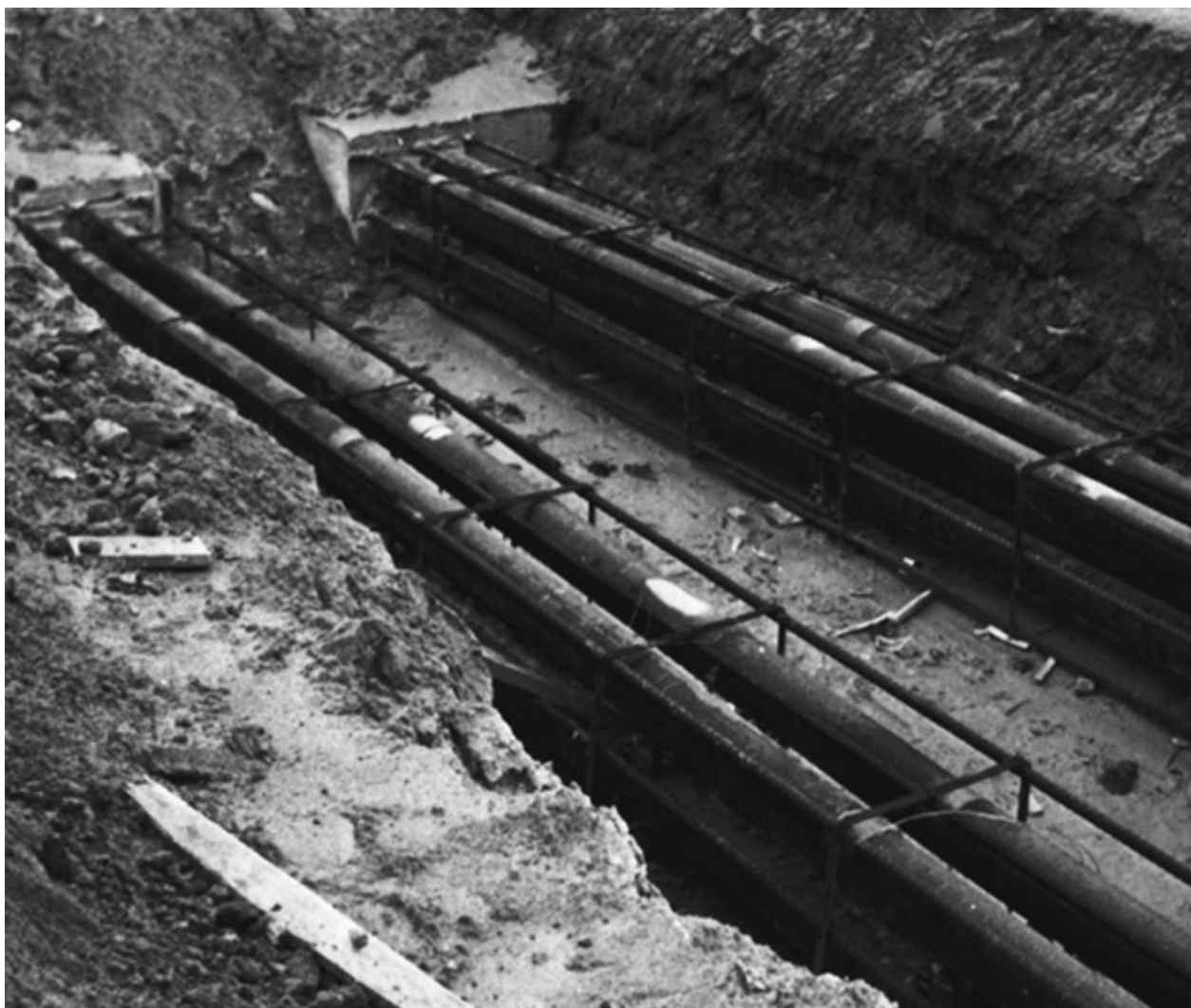
Fig. 352-5. All UL-listed rigid nonmetallic conduits are acceptable for use underground. PVC Schedule 40 and Schedule 80 do not require concrete encasement. Other types must observe UL and NEC rules on concrete encasement. (Sec. 352.10.)
