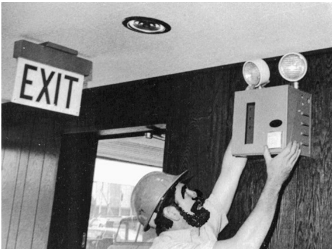
Fig. 700-1. Exit lights and wall-hanging battery-pack emergency lighting units are covered by Art. 700 whenever such equipment or provisions for emergency application are legally required by governmental authorities. (Sec. 700.1.)
