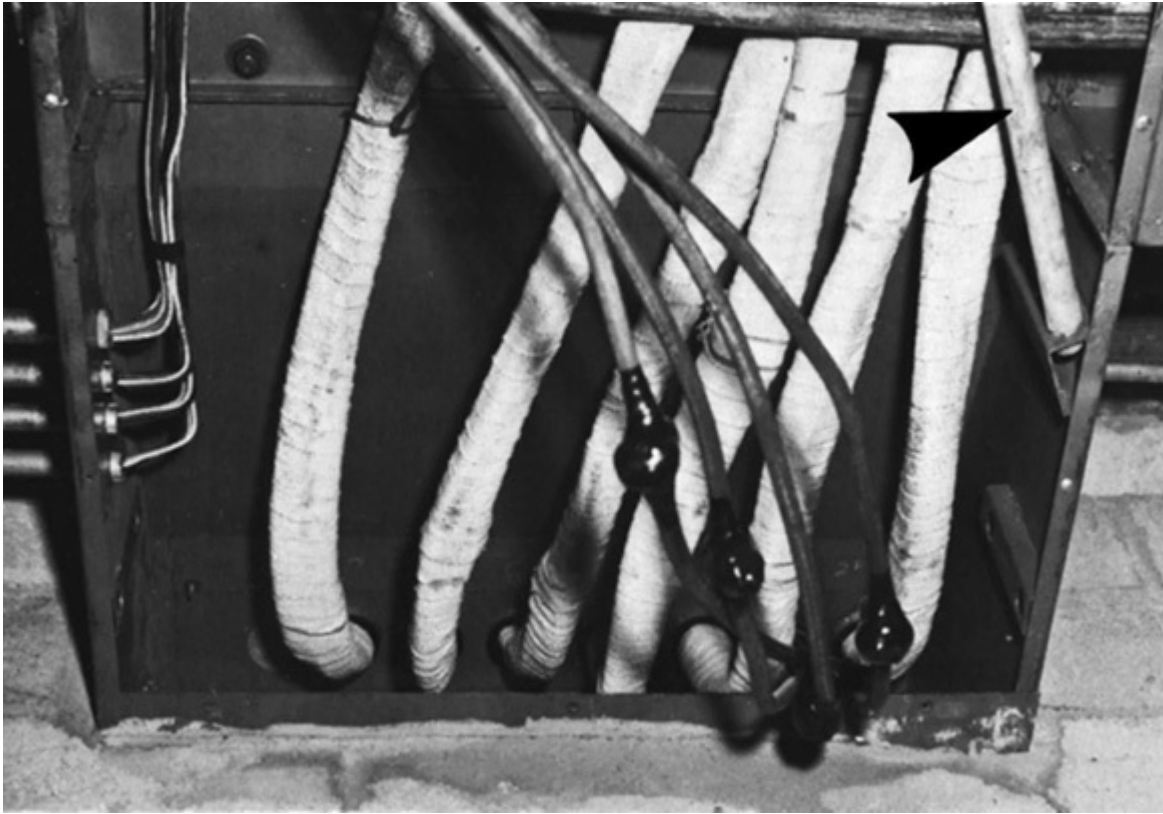
Fig. 314-39. If a pull box has any dimension over 6 ft (1.8 m), the conductors within it must be supported by suitable racking (arrow) or cabling, as shown here for arcproofed bundles of feeder conductors, to keep the weight of the many conductors off the sheet metal cover that attaches to the bottom of the box. (Sec. 314.28.)
