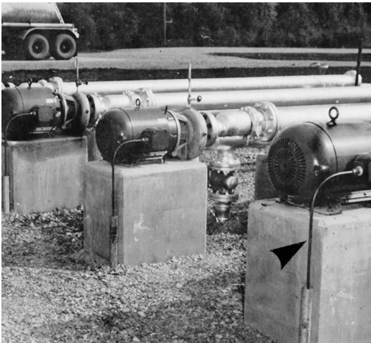
Fig. 332-2. Type MI is recognized for an extremely broad range of applications—for any kind of circuit, indoors or outdoors, wet or dry, and even in hazardous locations, as where MI motor branch circuits supply pumps in areas subject to flammable gases or vapors. (Sec. 332.10.)
