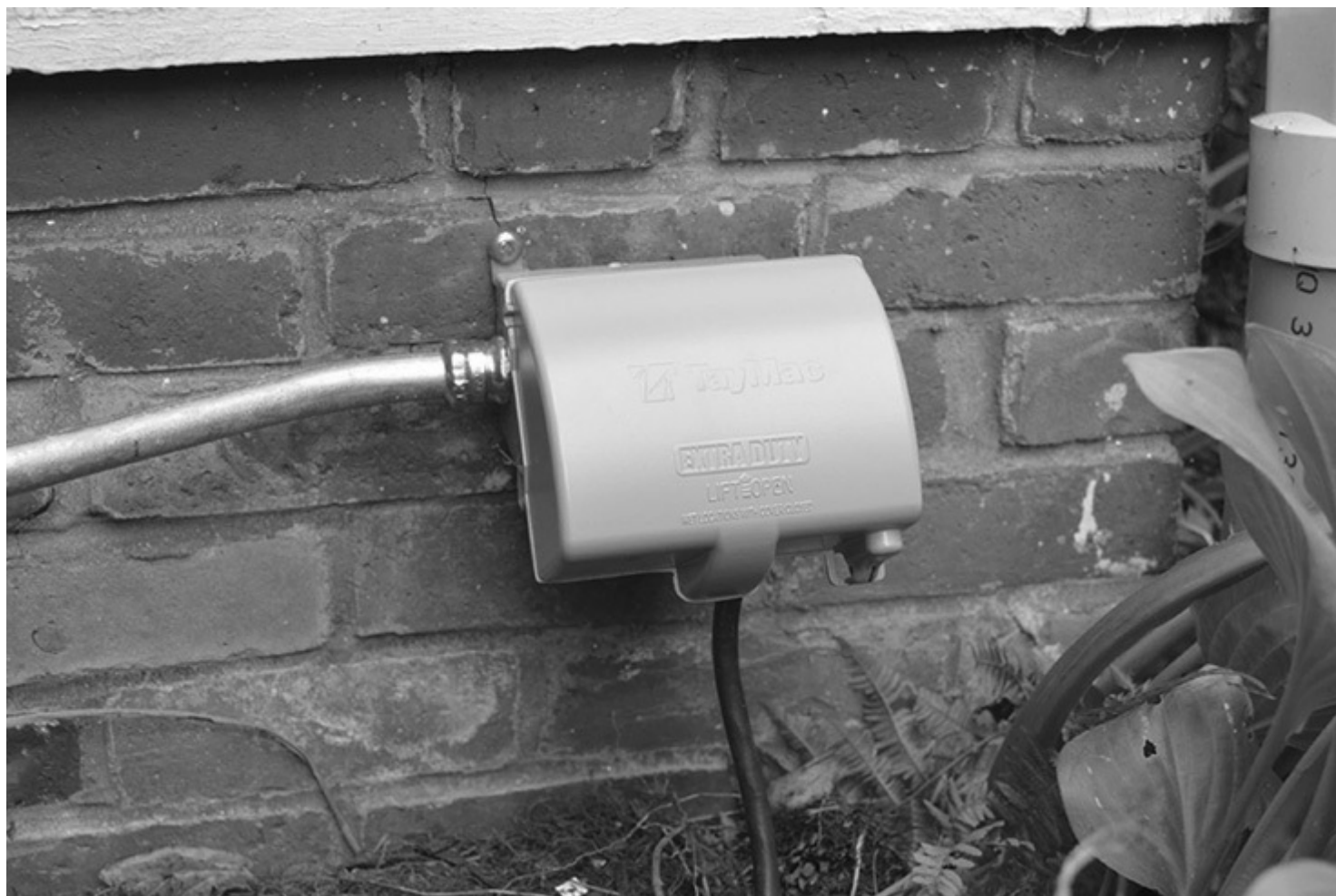
Fig. 406-7. A listed “outlet box hood” additionally identified as “extra duty.” This cover will protect the receptacle even when a cord-and plug-connected load is in use. (Sec. 406.9.)
