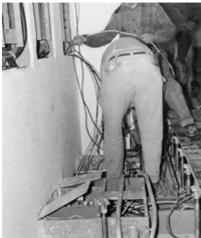
Fig. 645-2. Branch circuits from a panel-board to data processing receptacle outlets can be in a wide variety of Chap. 3 wiring methods. (Sec. 645.5.)
