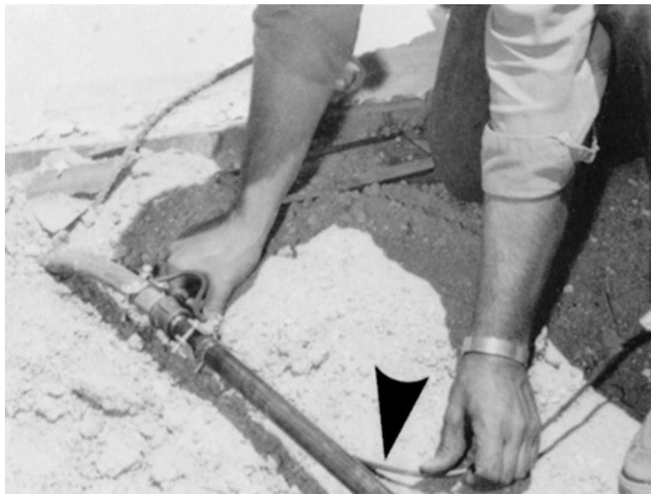
Fig. 680-13. 8 AWG insulated bonding conductors from several bonded items connect to the brass conduit, thereby using it as a bonding conductor. 680.26(B)(7) requires bonding of all “metal conduit” within 5 ft (1.5 m) of pool edge. (Sec. 680.26.)
