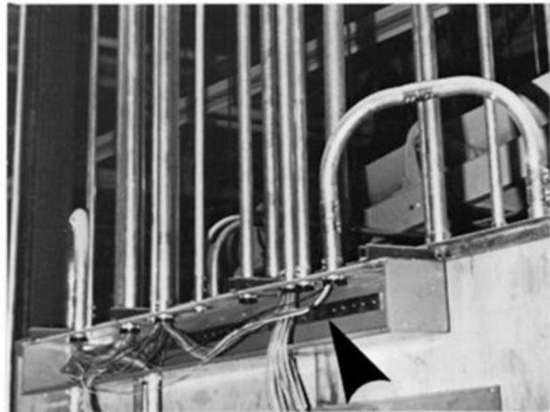
Fig. 366-1. Typical applications of auxiliary gutters provide the necessary space to make taps, splices, and other conductor connections involved where a number of switches or CBs are fed by a feeder (top) or for multiple-circuit routing, as at top of a motor control center (right) shown with a ground bus in gutter (arrow). (Sec. 366.1.)
