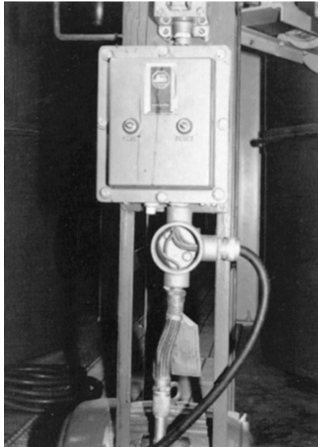
Fig. 501-13. Seal fitting of the round box type is used to seal the conduit run into the bottom of an explosionproof starter enclosure, with flexible fitting connection to the Class I, Division 1, Group D motor below and a watertight Class I cord connector control cable. (Sec. 501.15.)
