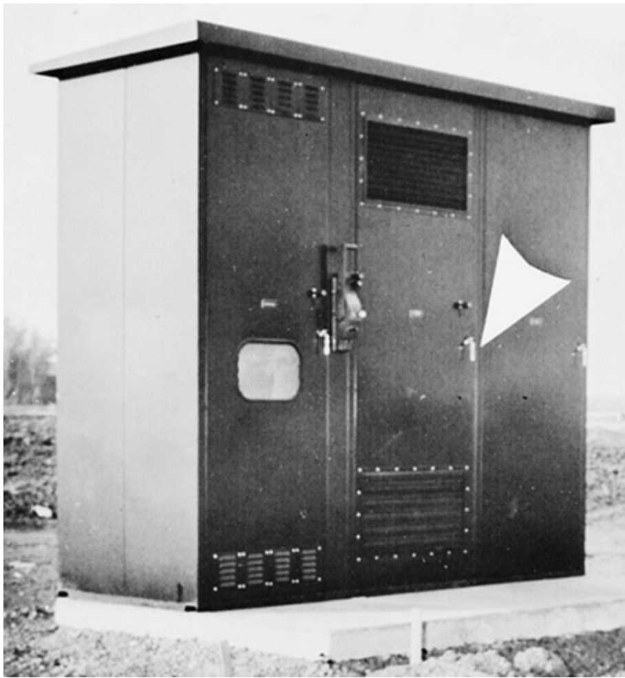
Fig. 110-27. Metal-enclosed high-voltage equipment accessible to the general public—such as pad-mount transformers or switchgear units installed outdoors or in indoor areas where the general public is not excluded—must have doors or hinged covers locked (arrow) if the bottom of the enclosure is less than 8 ft (2.5 m) above the ground or above the floor.
