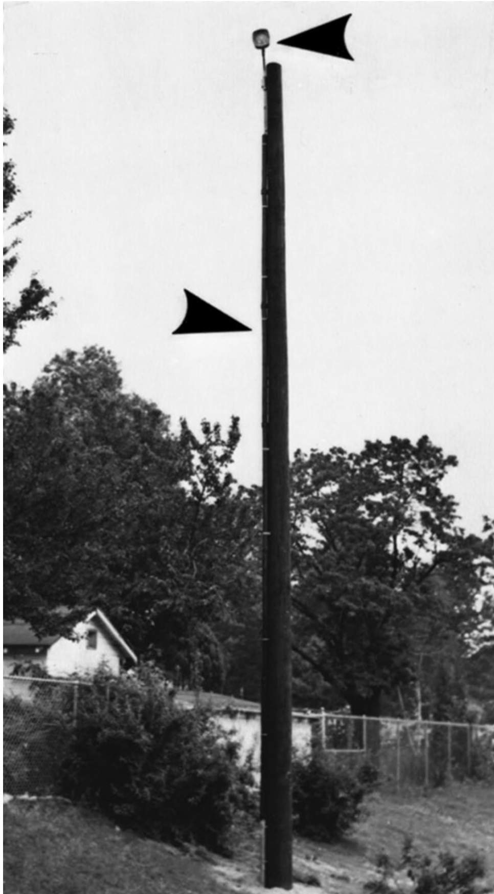
Fig. 352-2. PVC and RTRC conduits are the only rigid nonmetallic conduits that may be used
