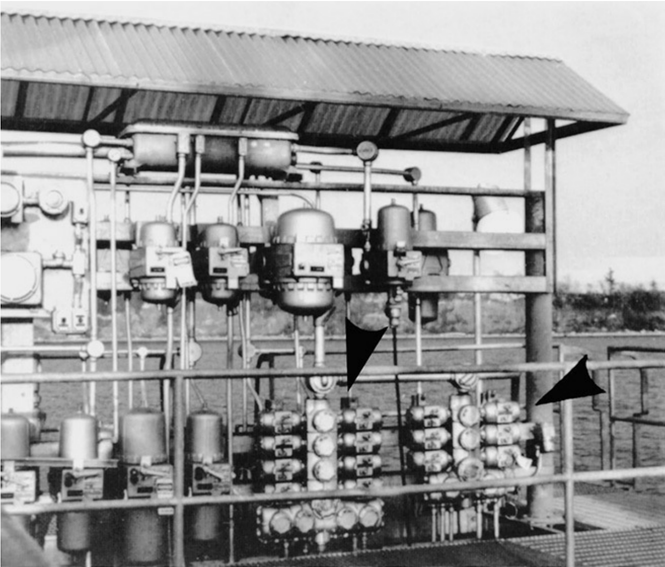
Fig. 501-31. Explosionproof panelboards (arrows) are assemblies made up of circuit-breaker housings coupled to wiring enclosures. Large explosionproof CB enclosure at center feeds the panelboards. Explosionproof motor controllers are at lower left. (Sec. 501.115.)
