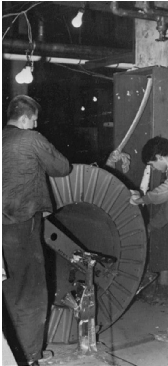
Fig. 590-8. A lampholder with a guard is proper protection for a lamp at any height in a temporary wiring system (above). Unguarded lamps at any height constitute a Code violation (right). (Sec. 590.4.)
