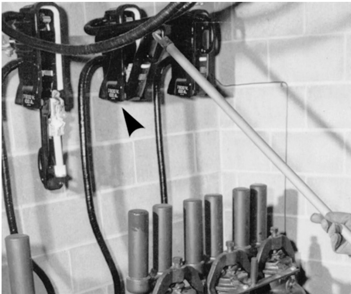
Fig. 490-7. Distribution cutouts are single-pole, fused, protective, and disconnect devices that are hook-stick-operable. Note voltage and current rating on case of each cutout (arrow), as required by part (C)(5) of 490.21. (Sec. 490.21.) The location appears to be indoors, and if so, would be controversial in light of the prohibition in 490.21(C)(1).
