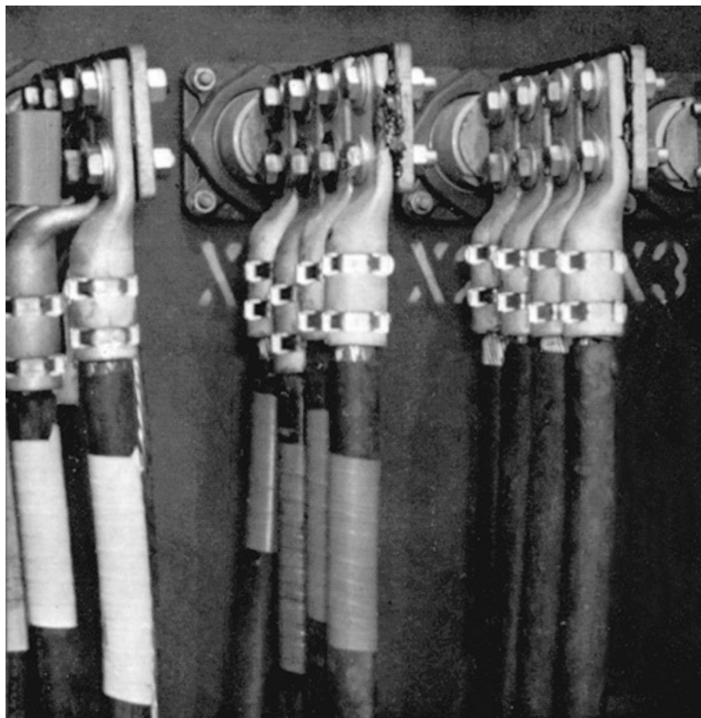
Fig. 200-3. Conductors of colors other than white or gray—in sizes larger than No. 6—may be used as grounded neutrals or grounded phase legs if marked white at all terminations—such as by white tape on the grounded feeder neutrals, at left. [Other color tapes are used on other circuit conductors to identify the three phases as A, B, and C—as required by 210.5(C) for branch circuits and 215.12(C) for feeders.] [Sec. 200.6(B).]
