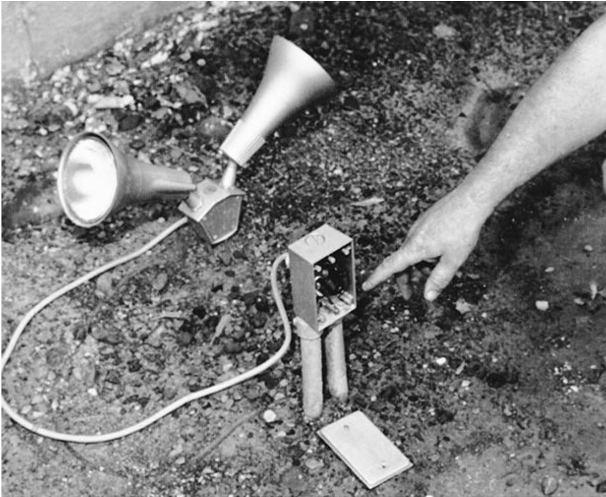
Fig. 400-2. This use of flexible cord to supply an outdoor lampholder assembly can readily be described as a “substitute for fixed wiring”—which is a prohibited use of cord. Here, the lampholders could have been attached to one or more threaded openings on an outlet box. (Sec. 400.12.)
