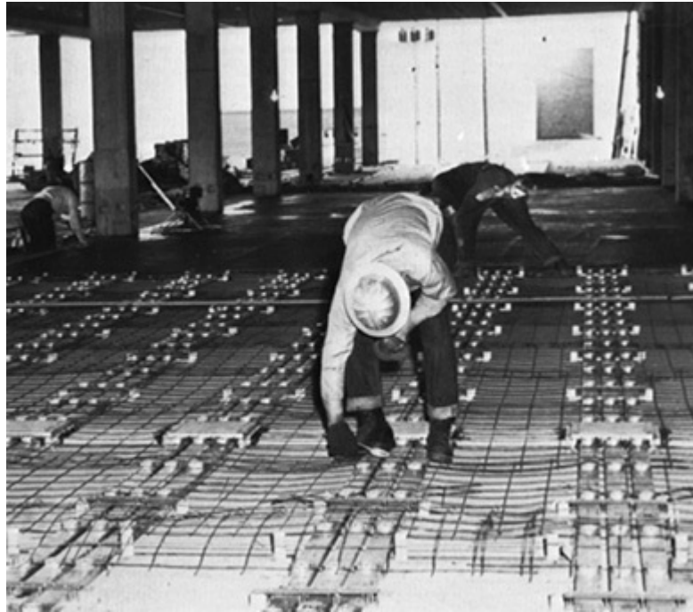
Fig. 390-1. Underfloor raceway system, with spaced grouping of three ducts (one for power, one for telephone, one for signals), is covered with concrete after installation on first slab pour. (Sec. 390.3.)
