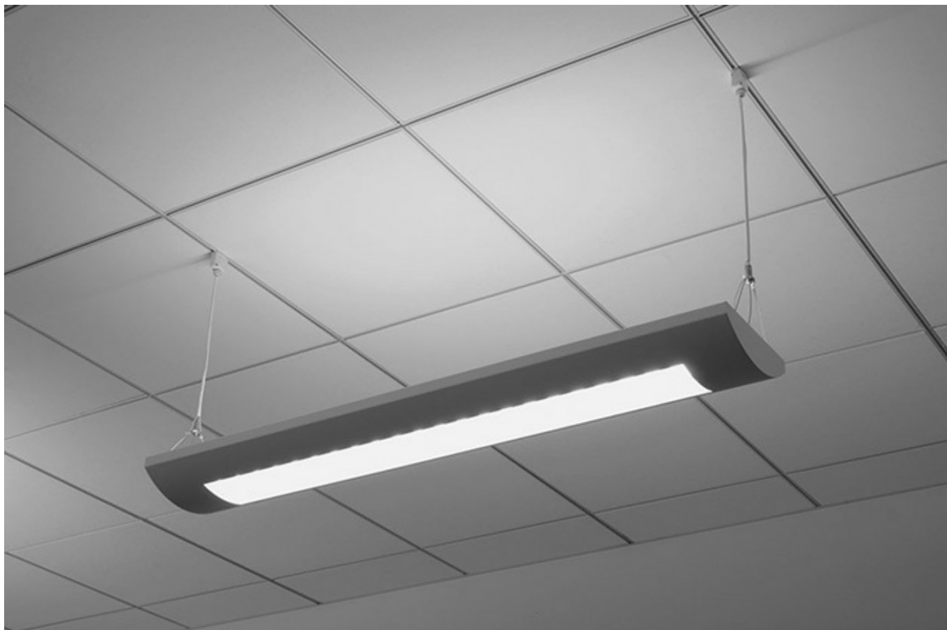
Fig. 393-2. This luminaire is fed from a pendant fitting that attaches to the inside of a specially constructed grid. [Sec. 393.40(A)(2)]. (Courtesy of EMerge Alliance®.)
