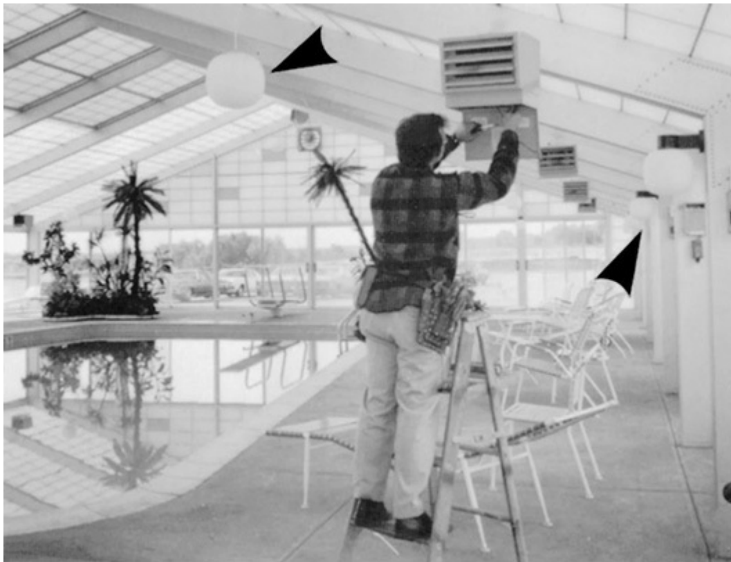
Fig. 680-7. The luminaires over the pool and for 5 ft (1.5 m) back from the edge must be at least 12 ft (3.7 m) above the maximum water level if their supply circuit is without GFCI protection. If GFCI
