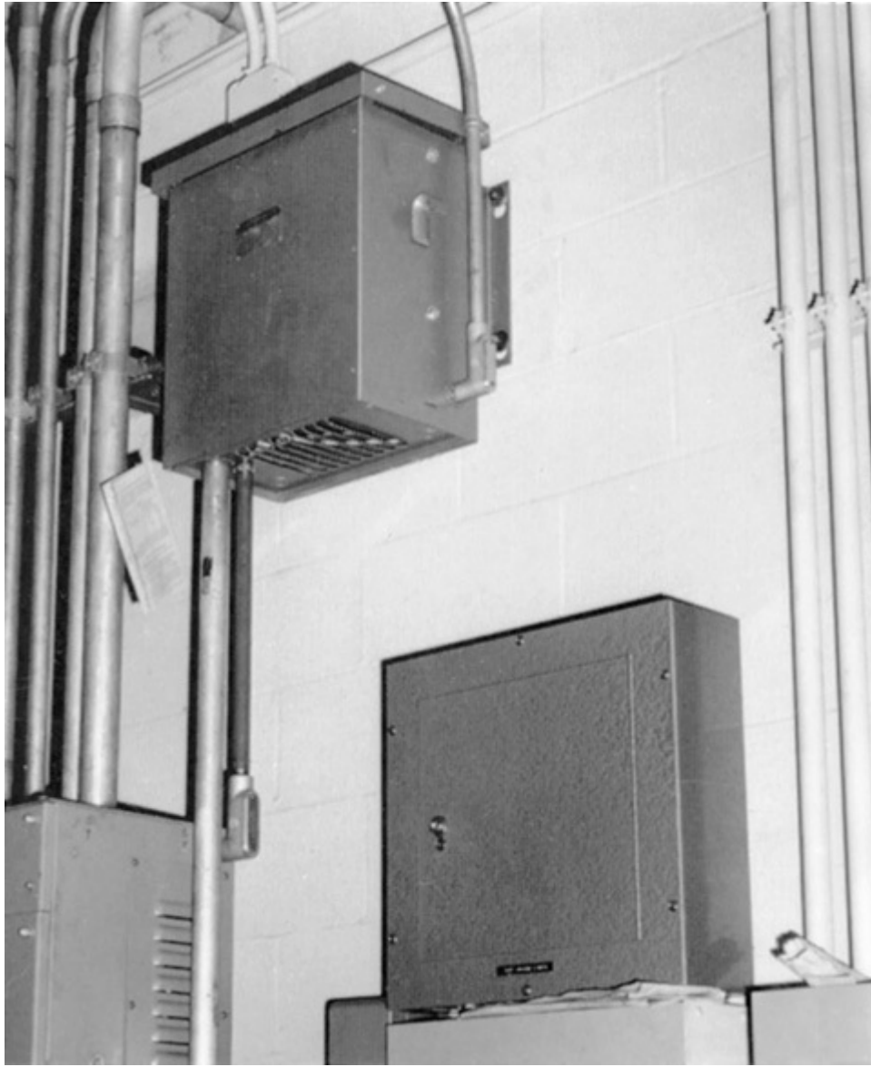
Fig. 450-24. Transformer mounted on wall (or suspended from ceiling) would be considered not readily accessible because a ladder would be needed to reach it. But, because it is “in the open,” such use conforms to 450.13(A). (Sec. 450.13.)
