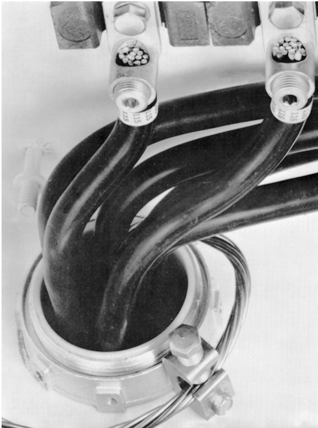
Fig. 517-5. Feeders to branch-circuit panelboards for critical care areas must be bonded. Figure 517-4 covers rules on grounding and bonding for the patient vicinity of a critical care area, with feeder conduit bonding as in this photo. [Sec. 517.19(D).]
