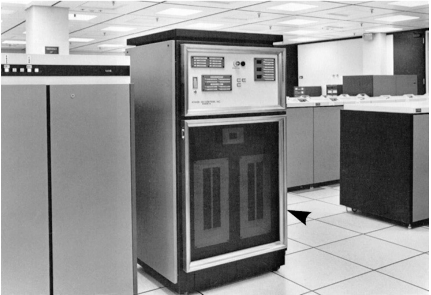
Fig. 645-5. Rapidly accelerating application of DP equipment in special DP rooms with wiring under a raised floor of structural tiles places great emphasis on Art. 645. “Computer power centers” (arrow) are complete assemblies for the supply of branch circuits to DP equipment, with control, monitoring, and alarm functions. (Sec. 645.10.)
