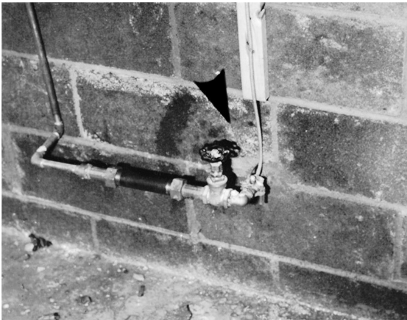
Fig. 250-33. Connection to an underground metal water-supply pipe is never adequate grounding for electric service equipment. (Sec. 250.53.)
