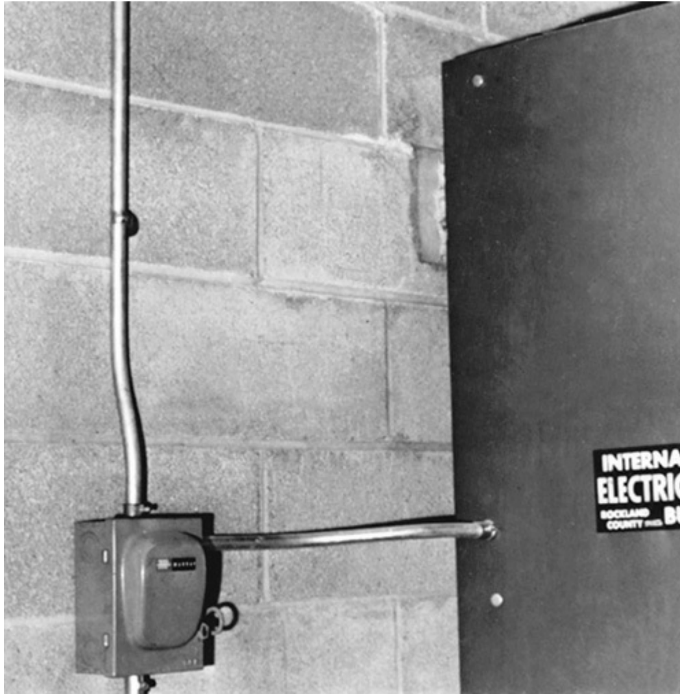
Fig. 230-34. Emergency disconnect close to service switchboard and fed by tap from it could readily be disabled by fault in board. (Sec. 230.72.)
