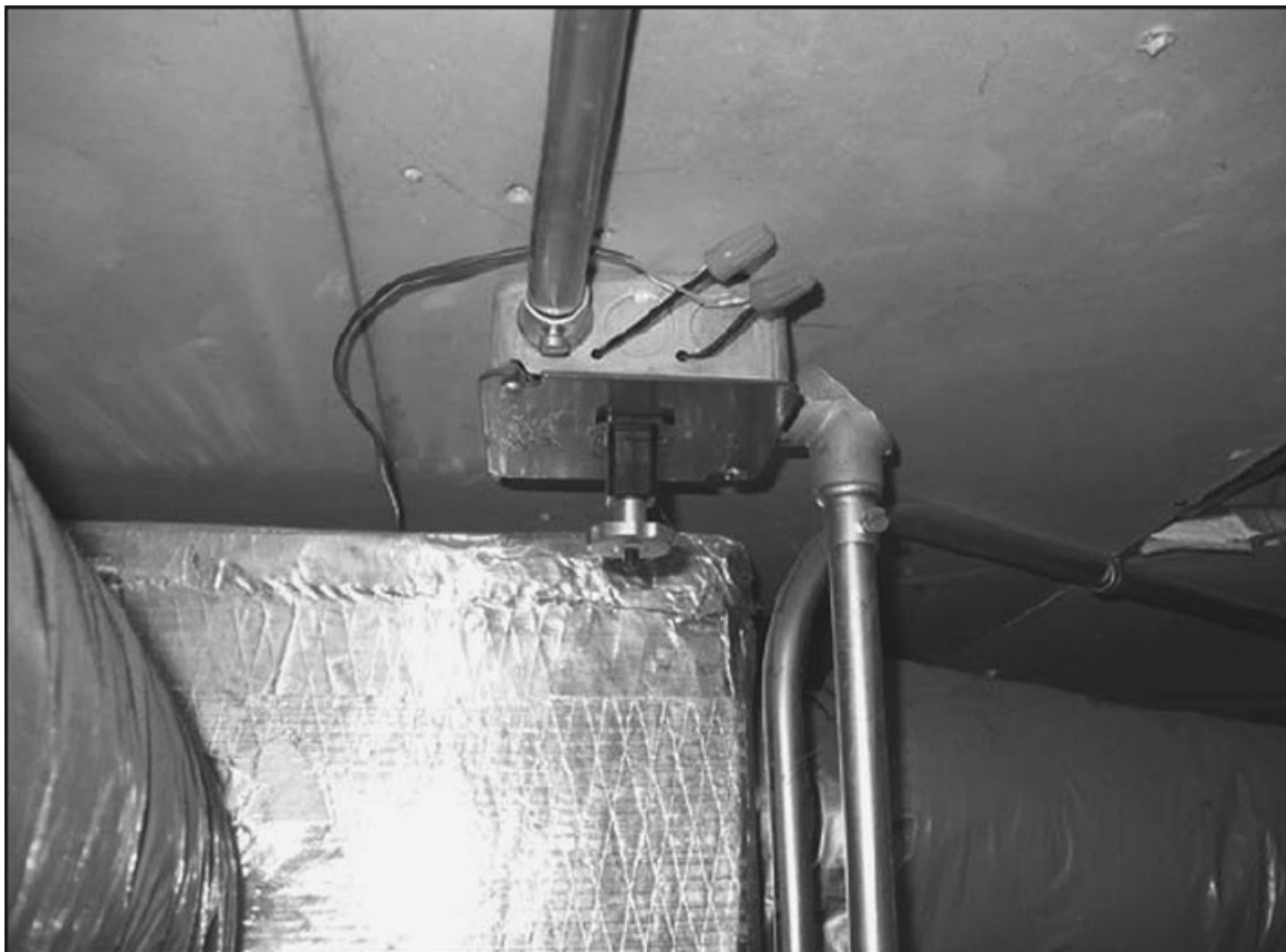
Fig. 300-1. The 14 AWG THHN leaving the box from the EMT riser and connected to 18-2 thermostat wire for a 24-V Class 2 circuit does comply with 300.3(C)(1), but violates 725.136(A).
