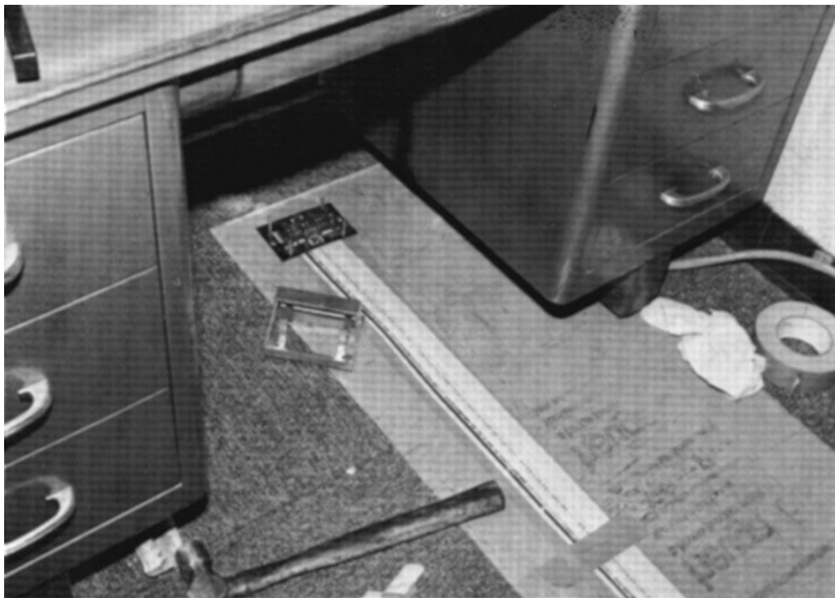
Fig. 324-1. Flat conductor cable (FCC) supplies terminal base for floor-outlet pedestal at exact location required for desk in office area. FCC is taped in position over an insulating bedding tape and then covered with a flat steel tape (not yet installed here) to protect the three conductors (hot leg, neutral, and equipment grounding conductor) in the flat cable. Carpet squares are used to cover the finished cable runs.
