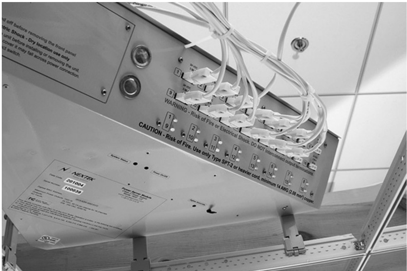
Fig. 393-3. This power supply will supply 16 separate grid lines, which the manufacturer estimates will cover between 800 and 1000 sq. ft of ceiling. The listing mark is just visible at the opposite corner. [Sec. 393.6(B)(2).] (Courtesy of EMerge Alliance®.)
