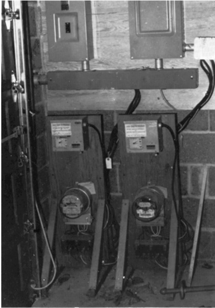
Fig. 590-2. Temporary wiring techniques are permitted for 90 days for such “experimental” work as energy demand analysis. (Sec. 590.3.)
