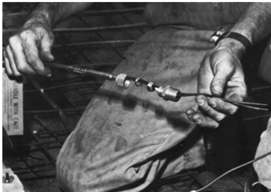
Fig. 332-3. Termination fitting for Type MI cable must be an approved connector, with its component parts assembled in proper sequence. [Sec. 332.40(A).]
