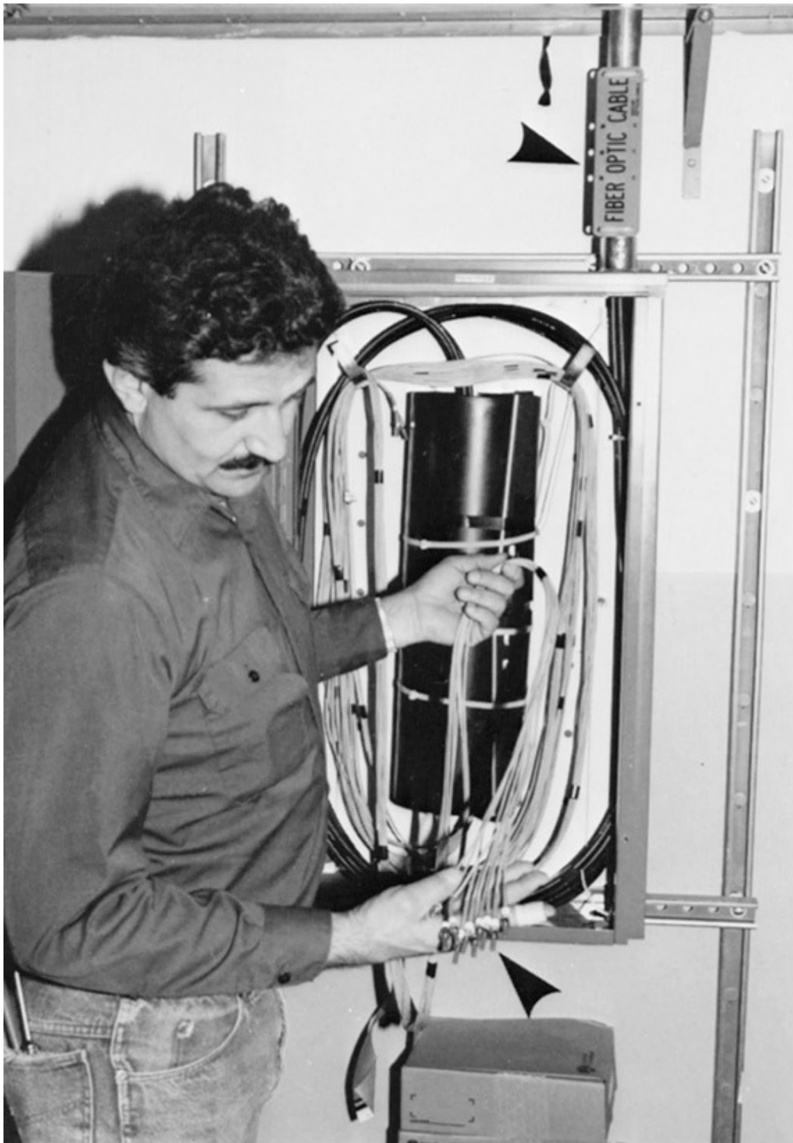
Fig. 770-4. A NEMA 3R splice box in the telecommunications room of one of the buildings, with two 10-conductor cables entering at top (arrow) and the individual FO conductors terminated in special connectors (bottom arrow). FO conductors are used as data communication links between five different buildings in which a banking firm has branch locations in a large city. The overall circuiting includes the runs within the buildings (connecting to computers, video equipment, telephones, and telecommunications equipment) and over 5 mi of underground 30-conductor FO cable with a metal armor sheath run under the city in ducts.
