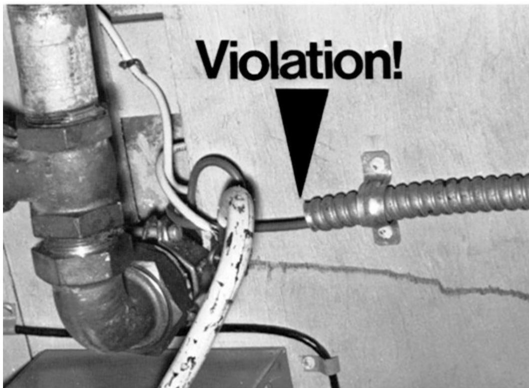
Fig. 250-56. Two examples of very clear violations of the rule that requires enclosing metal raceways (rigid metal conduit at top and flex at right) to be bonded at both ends to a grounding electrode conductor within the raceway. [Secs. 250.92 and 250.64(C).]
