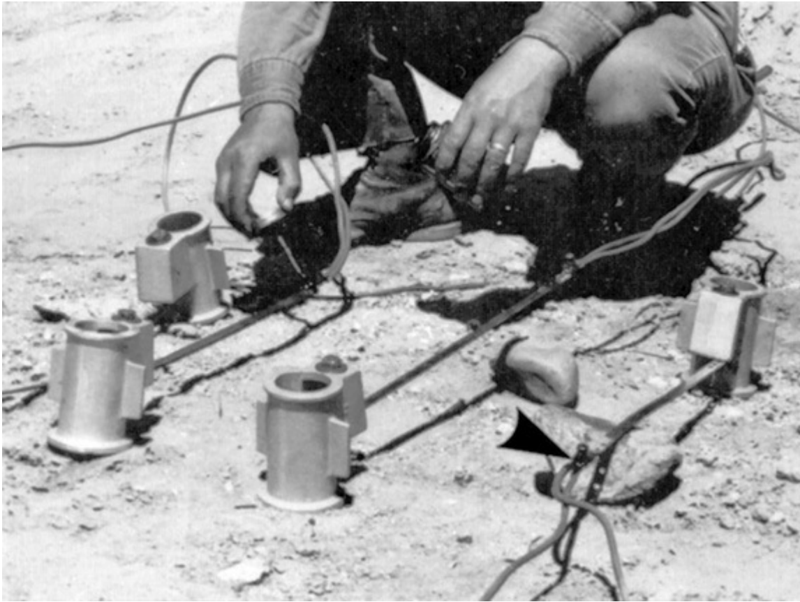
Fig. 680-16. Fittings for pool ladders have bonding strips attached to them for connection of the No. 8 bonding conductor. When the supports are set in the concrete deck, the bonding connections tie them all together. The 8 AWG bonding connections are shown (arrow) and a protective coating is painted on the connectors to protect against corrosion. (Sec. 680.26.)
