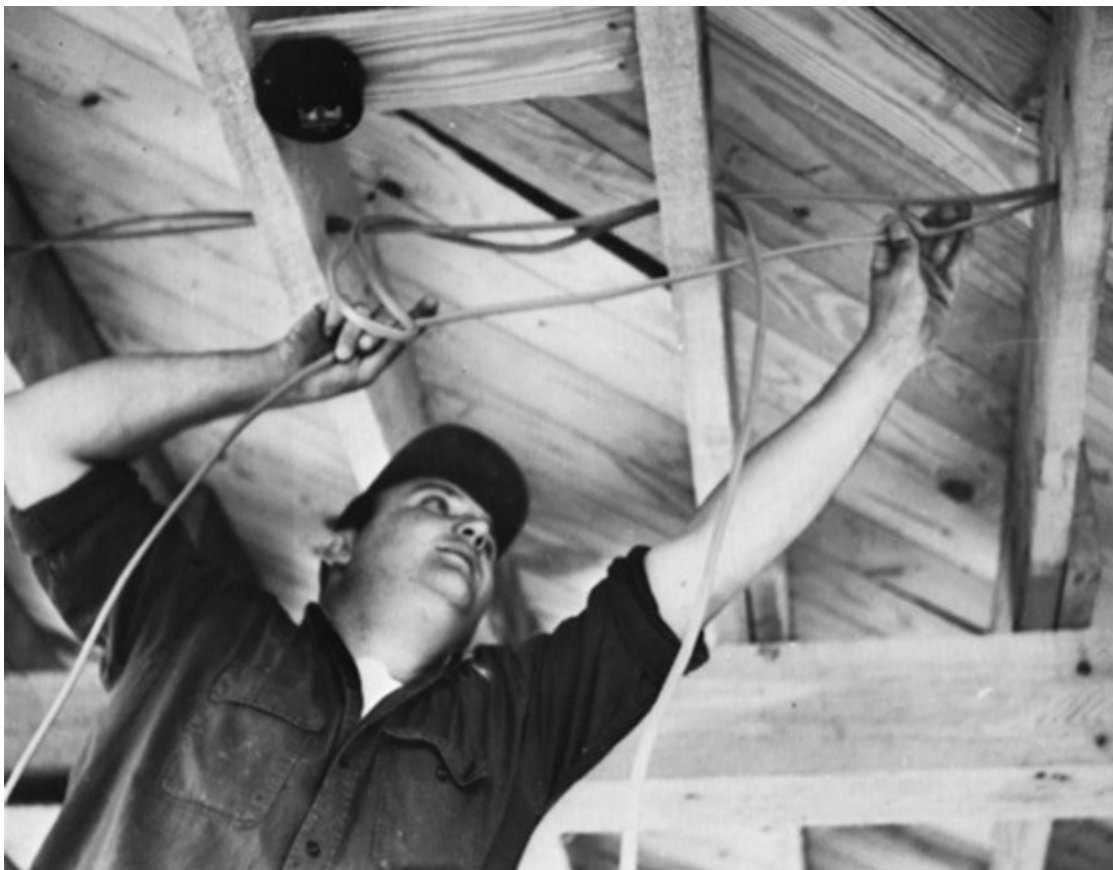
Fig. 300-47. A joist space through which Type NM cable passes “perpendicular to the long dimension” of the space may be closed in to form a duct-like space for the cold-air return of a hot-air heating system—but only in a “dwelling unit.”
