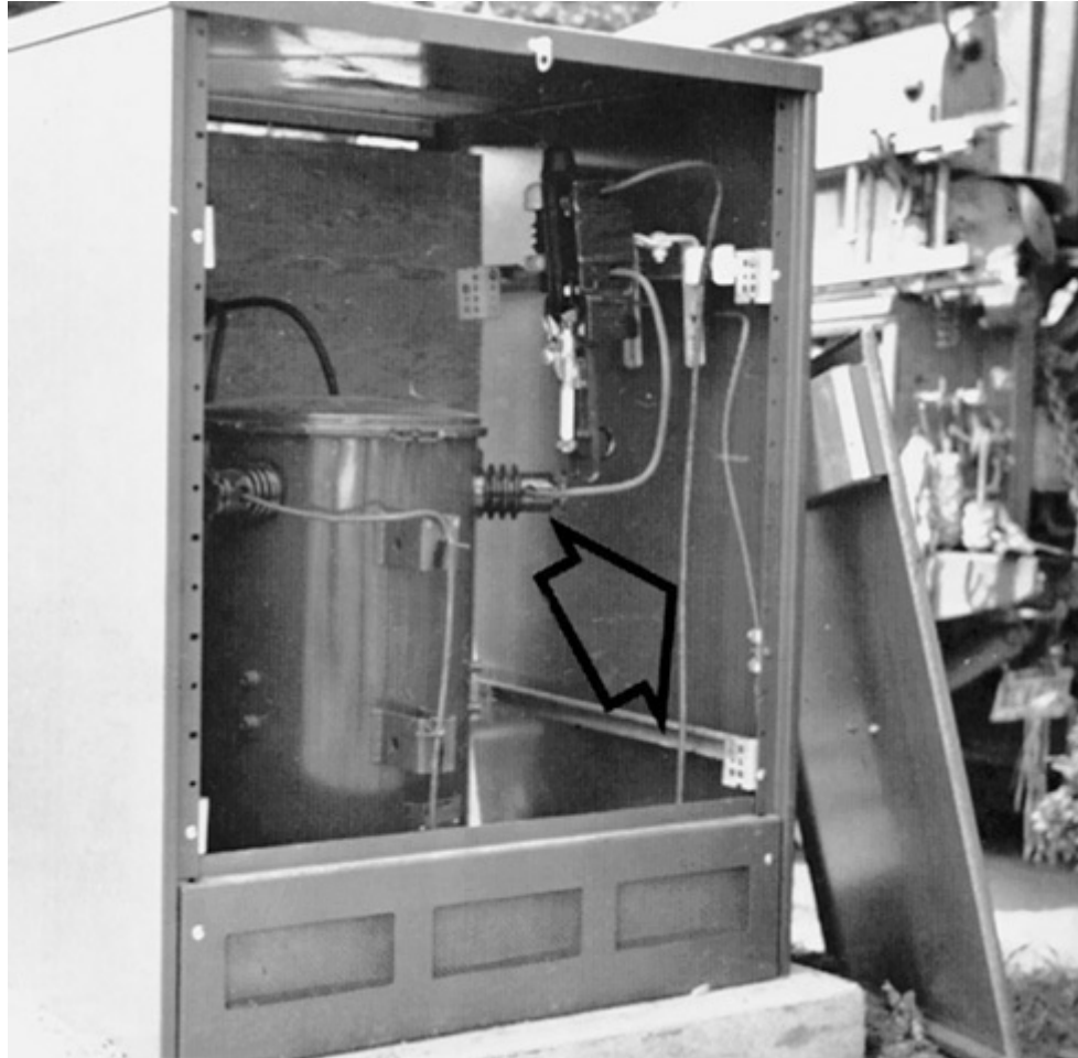
Fig. 310-1. A nonshielded conductor (arrow) is permitted for use on a 2300-V circuit (phase-to-neutral), as shown here, only if the conductor is listed by UL or another national test lab and approved for use without electrostatic shielding. [Sec. 310.10(E).]
