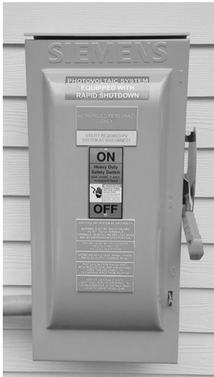
Fig. 690-4. The switch (shown in the open position) is the PV system disconnecting means. The utility (in this jurisdiction) required an open blade, outside mounted switch, connected ahead of the service equipment [permitted by 230.82(6)]. The switch is also wired as the rapid shutdown initiation device. Although installed under the 2014 NEC , the labeling largely meets the intent of 690.56(C) (3), although it misses the \frac{3}{8} -in. height rule. The labeling does comply with the 2017 NEC with respect to its system disconnecting function [690.13(B)]. Courtesy, Solar Design Associates, Inc.
