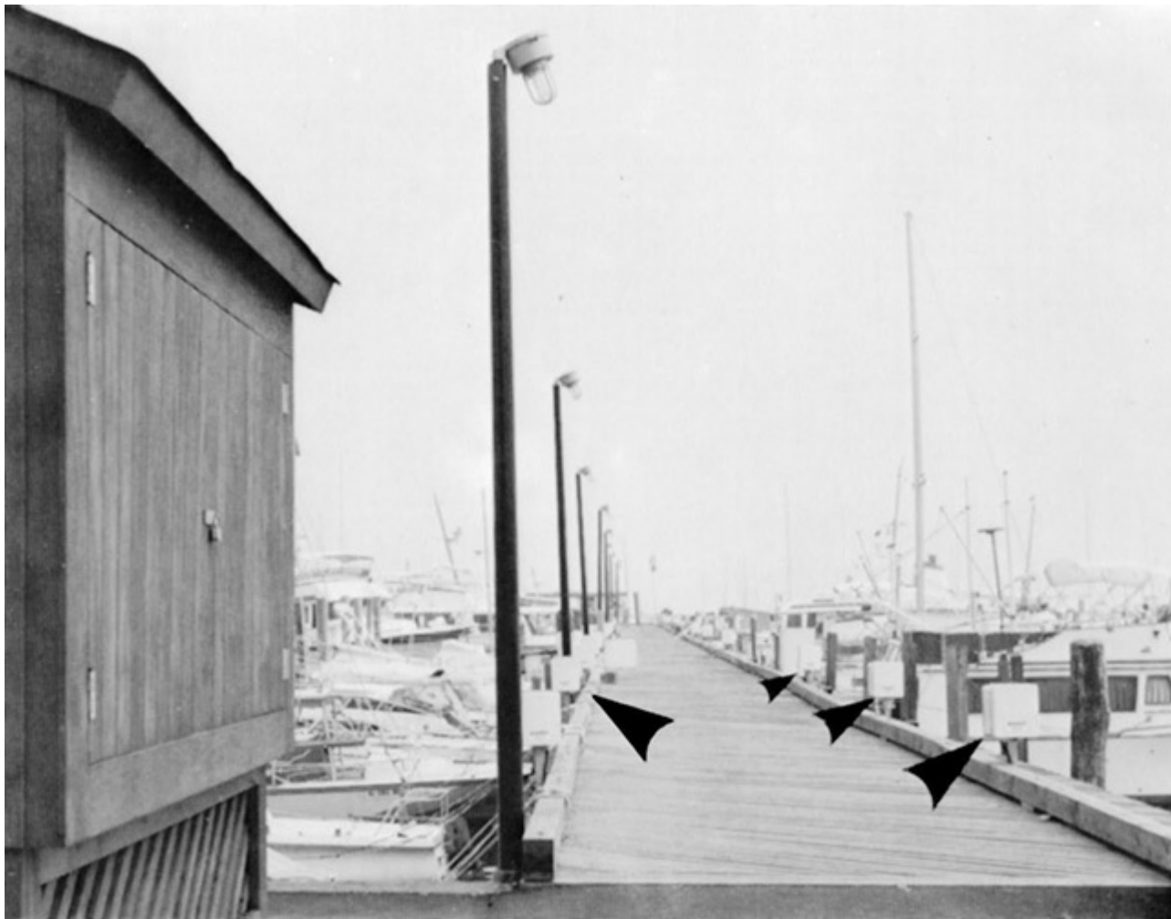
Fig. 555-1. This is one part of a 406-boat marina where shore power is supplied to moored boats from receptacle power pedestals (arrows) supplied by cables run under the pier from a panelboard in the shed at the left. (Sec. 555.1.)
