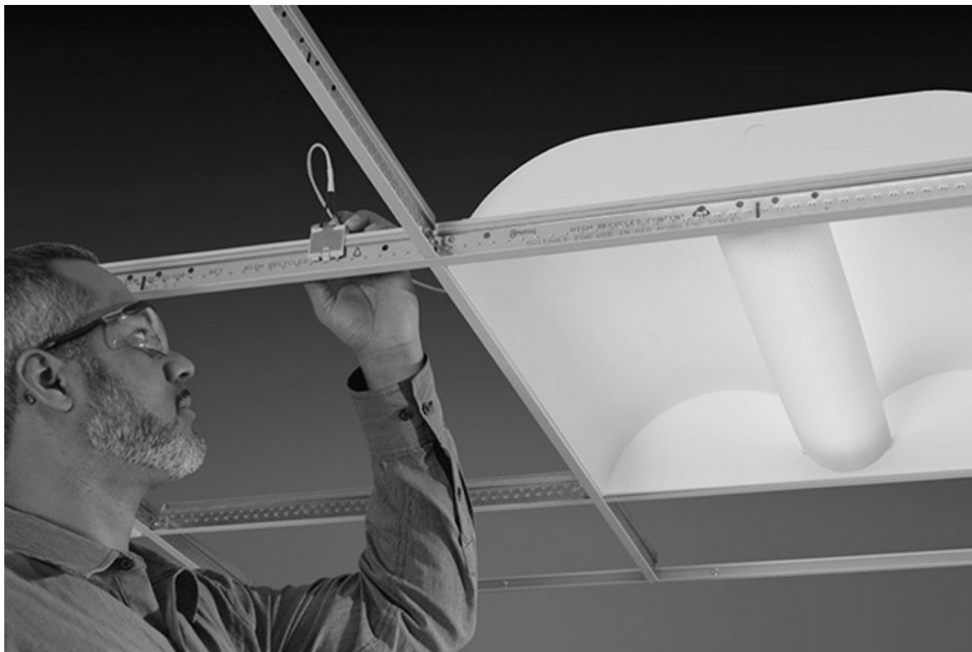
Fig. 393-1. The top of this T-bar has a conductor running on both sides of it carrying a Class 2 circuit accessible through the fitting being installed in the photo to supply the luminaire. [Sec. 393.40(A)(1).] (Courtesy of EMerge Alliance®.)
