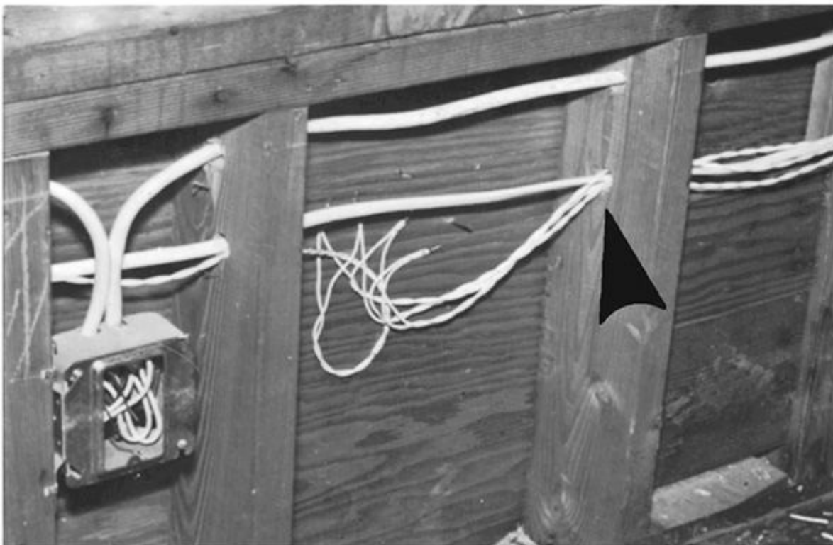
Signal and alarm wiring is run through the same stud holes as the NM cables. The NEC does not prohibit use of more than one cable through a single hole.
