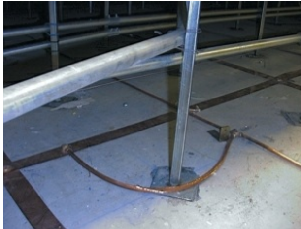
Photo 18.4 Signal reference grid connections independent of floor supports using 2" wide copper strips in a 2' x 2' pattern
