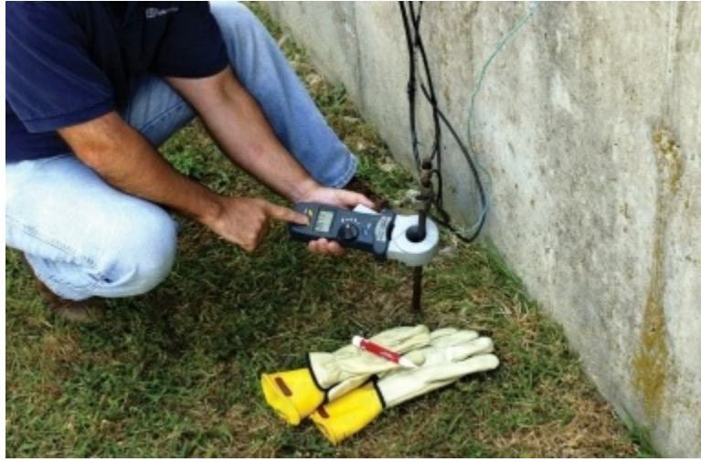
Photo 6.5 Clamp-on test instrument being used to test a facility grounding electrode Courtesy of Megger
