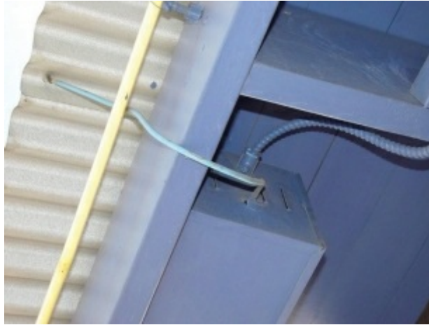
Photo 16.6 Violation shows metal parts of a structure being used as a neon secondary (high voltage) return circuit to transformer. There are numerous other violations in the photo as well.
