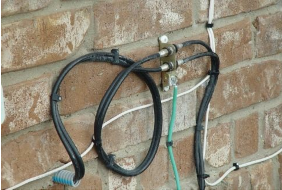
Photo 19.3 Coaxial cable shields grounded at point of entrance to building or structure
