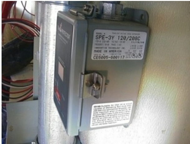
Photo 18.7 Surge protective device (SPD) labels
