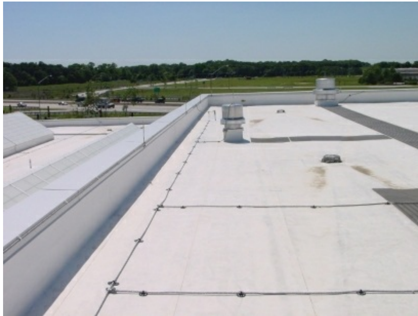
Photo 21.4 Example of air terminal spacing on roof showing air terminal spacing within 600 mm (2 ft) of the edge and at a spacing of 6.0 m (20 ft) around the perimeter Courtesy of Lightning Prevention Systems of West Berlin, NJ
