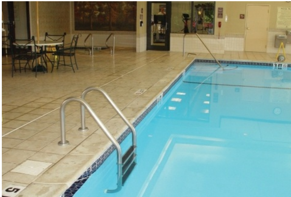
Photo 16.10 A stainless steel handrail provides the bonding means for the pool water.
