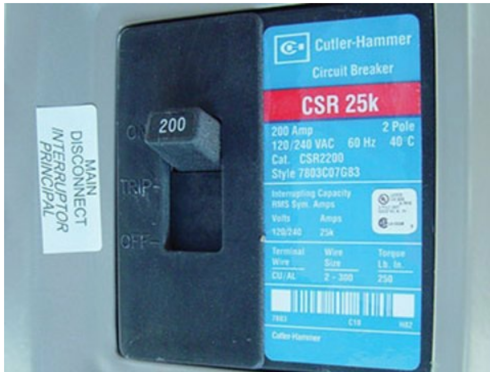
Photo 3.3 Breaker with slash voltage rating (120/240 V)
