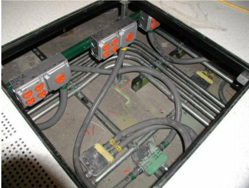
Photo 18.3 Isolated grounding receptacles installed under a raised floor in an information technology (IT) room
