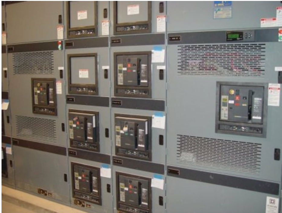
Photo 14.8 Residual GFPE equipment (breaker-types) in a switchboard
