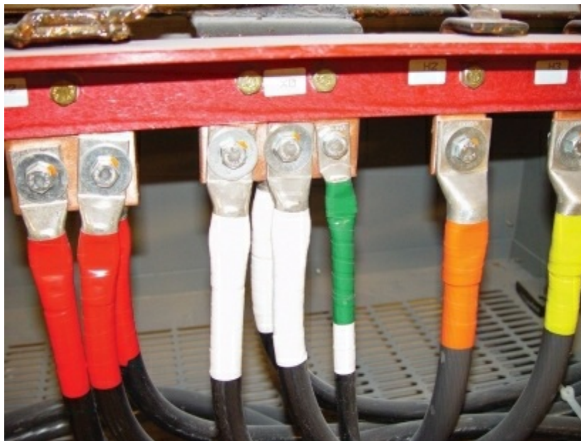
Photo 12.2 System bonding jumper in source enclosure
