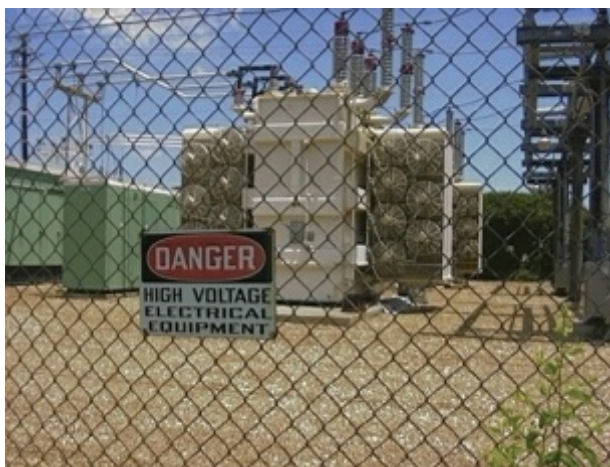
Photo 20.2 Substation surrounded by a grounded chain-link fence
