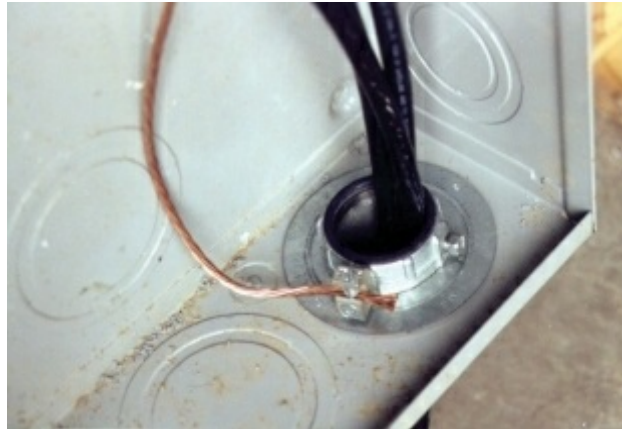
Photo 8.5 Bonding around reducing washers at coated enclosures to maintain continuity and the capacity to conduct any fault current that might be imposed. Bonding around reducing washers is always required when raceways contains service conductors (at any voltage).
