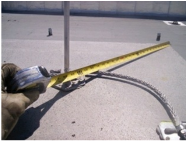
Photo 21.3 Measurement to ensure air terminal is no greater than 600 mm (2 ft) from corner of roof Courtesy of Bonded Lightning Protection of Argyle, TX
