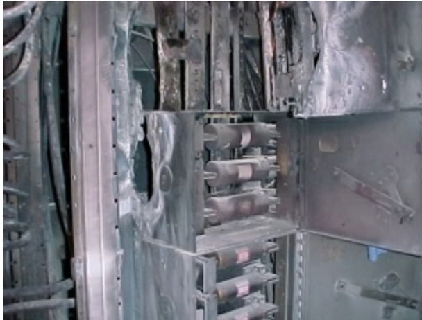
Photos 14.4 and 14.5 This equipment endured an arcing event that resulted in extensive destruction (an arcing burn down) of the equipment. GFPE could have prevented, or at least limited, this amount of damage.
