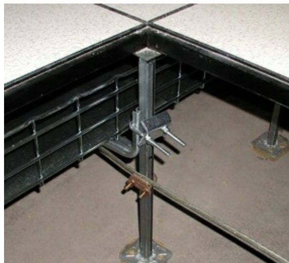
Photo 18.5 Raised floor platform structure used as a signal reference grid
