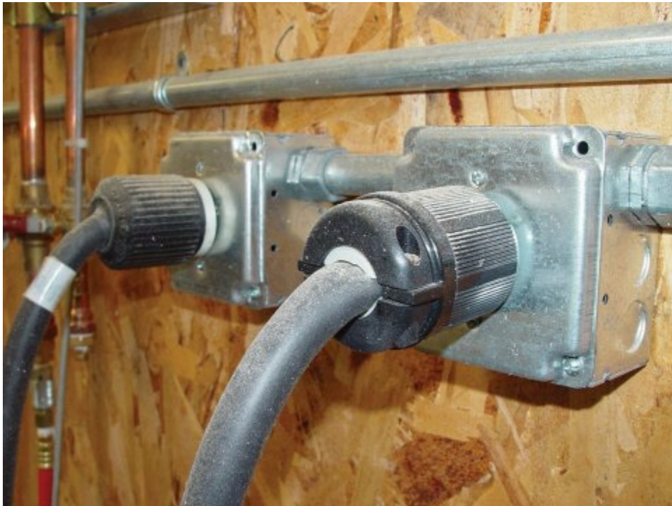
Photo 8.6 Surface-mounted box with raised cover and receptacle
