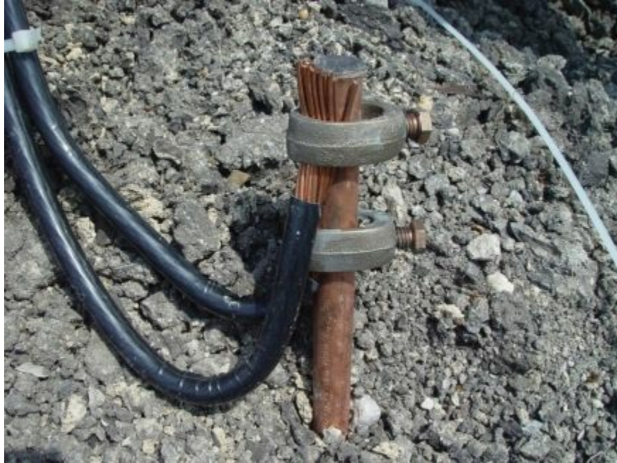
Photo 6.1 Grounding electrode (iron core, copper-clad rod type)
