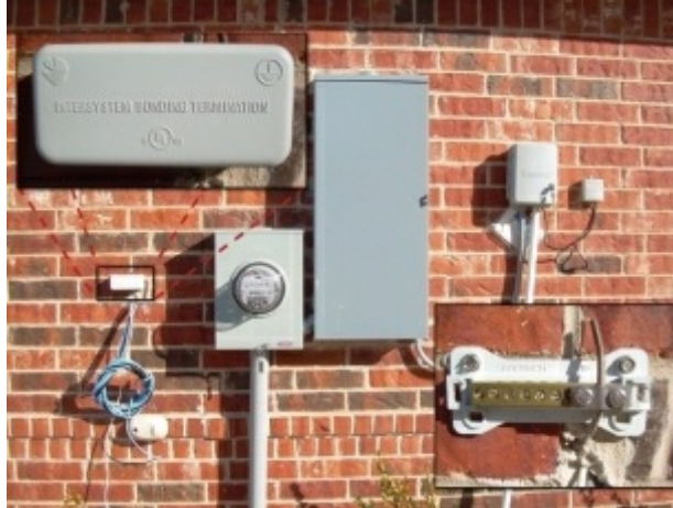
Photo 19.2 Communications system grounding electrode conductor connected to intersystem bonding termination
