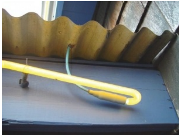
Photo 16.7 Violation shows a connection from the last tubing electrode to the metal parts of a structure used as the high voltage secondary return to the neon transformer. There are numerous other violations in the photo as well.
