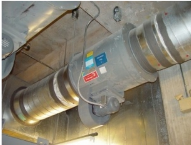
Photo 9.2 Equipment grounding conductor is installed to ground and bond electrical equipment. Exhaust fan motor is shown and equipment grounding conductor is installed in flexible metal conduit.
