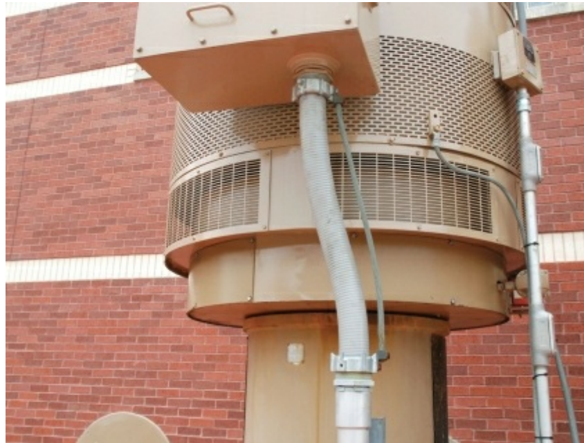
Photo 8.8 Equipment bonding jumper outside raceway
