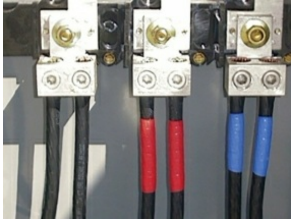
Photo 2.2 Ground faults rarely occur at bolted connections
