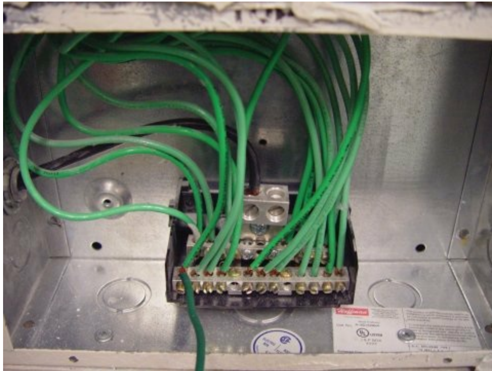
Photo 15.2 Patient equipment grounding point [517.19(E)]
