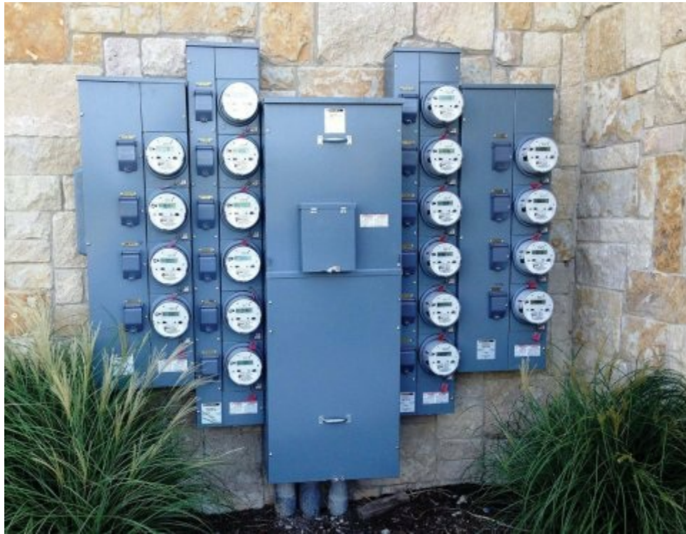
Photo 9.9 Meter equipment enclosures installed immediately adjacent to disconnecting means
