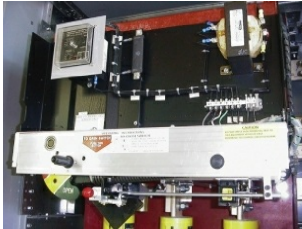
Photos 14.6 and 14.7 GFP equipment (bolted pressure switch with GFPE)
