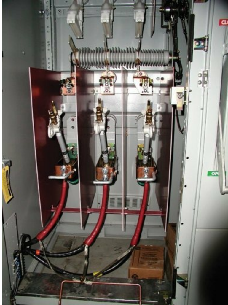
Photo 20.3 15,000-volt cables terminated at a switch showing stress reduction means and bleed wires connected to ground (earth)
