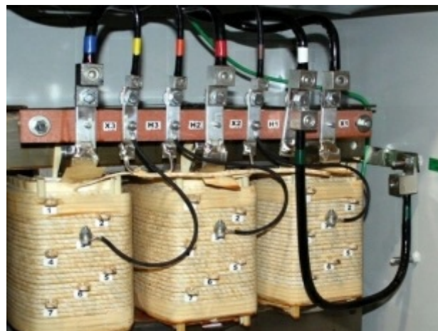
Photo 12.1 Transformer-type separately derived system
