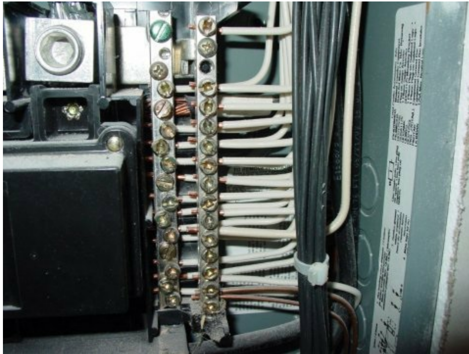
Photo 10.4 Grounded conductor terminal bar showing only one wire per terminal connected
