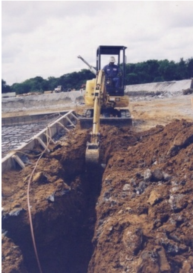
Photo 21.13 Installation of a ground ring electrode Courtesy of East Coast Lightning Equipment of Winsted, CT
