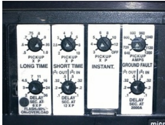
Photo 14.10 GFPE setting adjustments (breaker-type)
