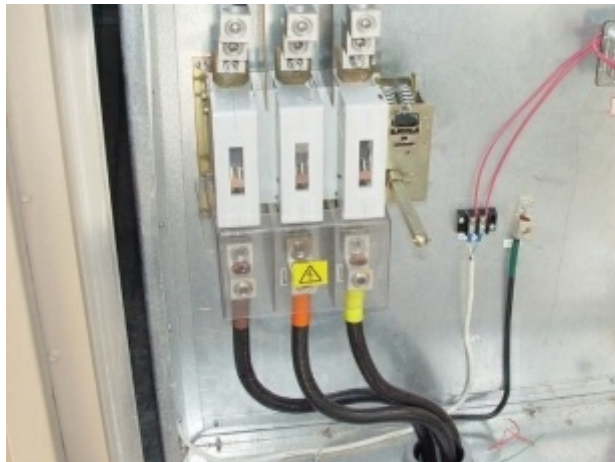
Photo 9.1 Equipment grounding conductor connected to equipment enclosure
