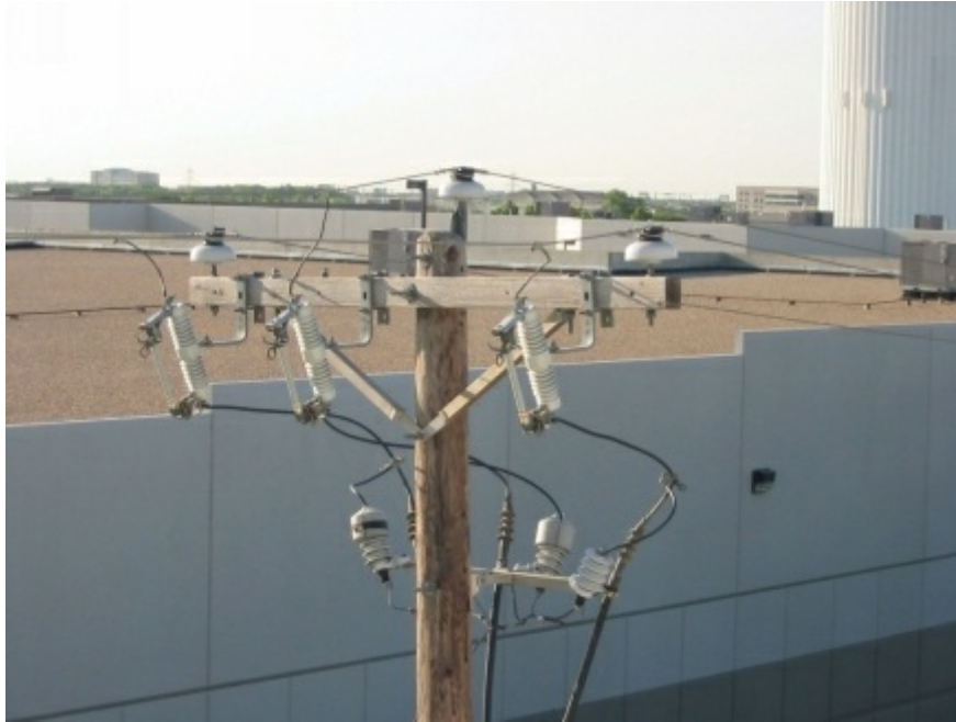
Photo 20.1 High voltage lines typically connected to surge arresters at pole locations
