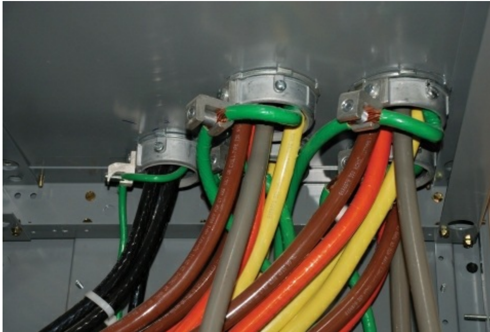
Photo 9.7 Equipment grounding conductors in each raceway of parallel feeder
