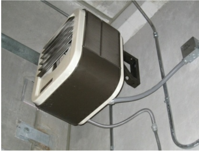
Photo 9.3 Flexibility necessary after installation (for aiming heater)
