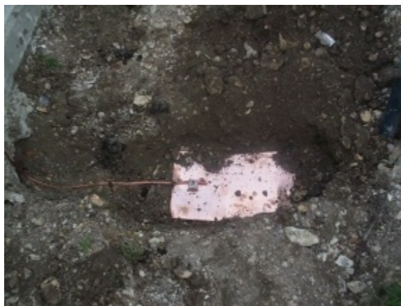
Photo 21.12 Example of a buried copper plate grounding electrode Courtesy of Bonded Lightning Protection of Argyle, TX
