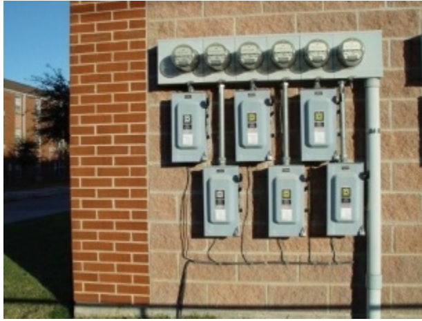
Photo 7.1 Common grounding electrode conductor and taps
