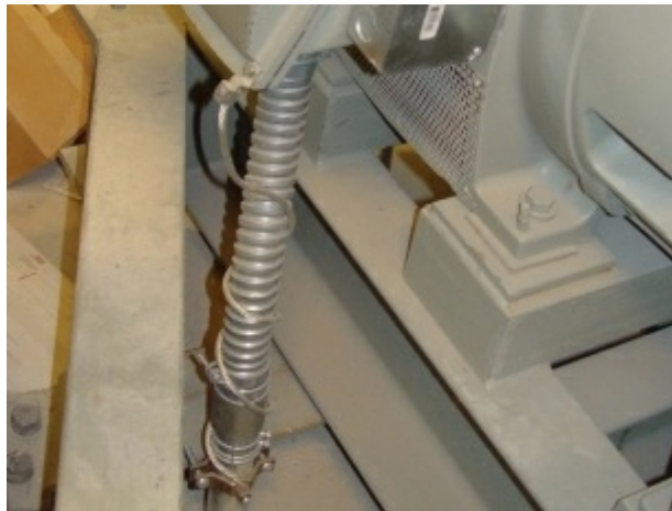
Photo 10.1 Equipment bonding jumper installed outside of flexible metal conduit [less than 1.83 m (6 ft)]
