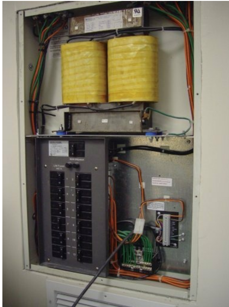
Photo 15.3 Isolated power systems equipment
