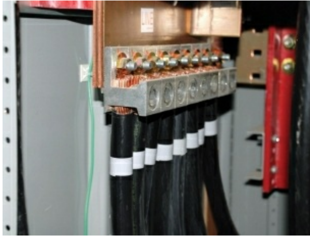
Photo 3.1 Grounded neutral conductor identification
