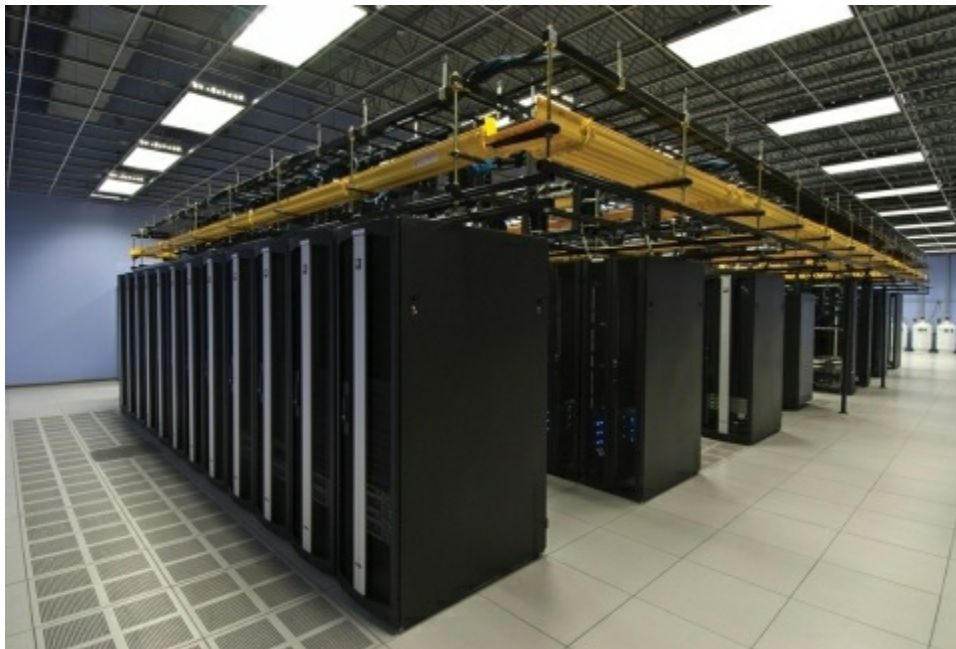
Photo 18.1 Information technology equipment
