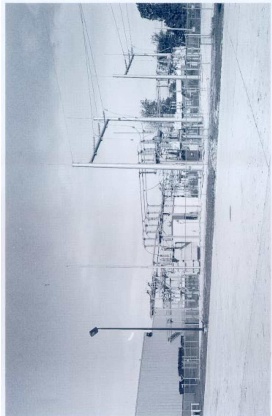
Figure 15-1 —An industrial substation
