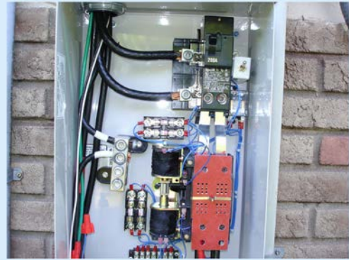
Standby System Capacity - Automatic Transfer Equipment 702.4(B)(2)(a)
